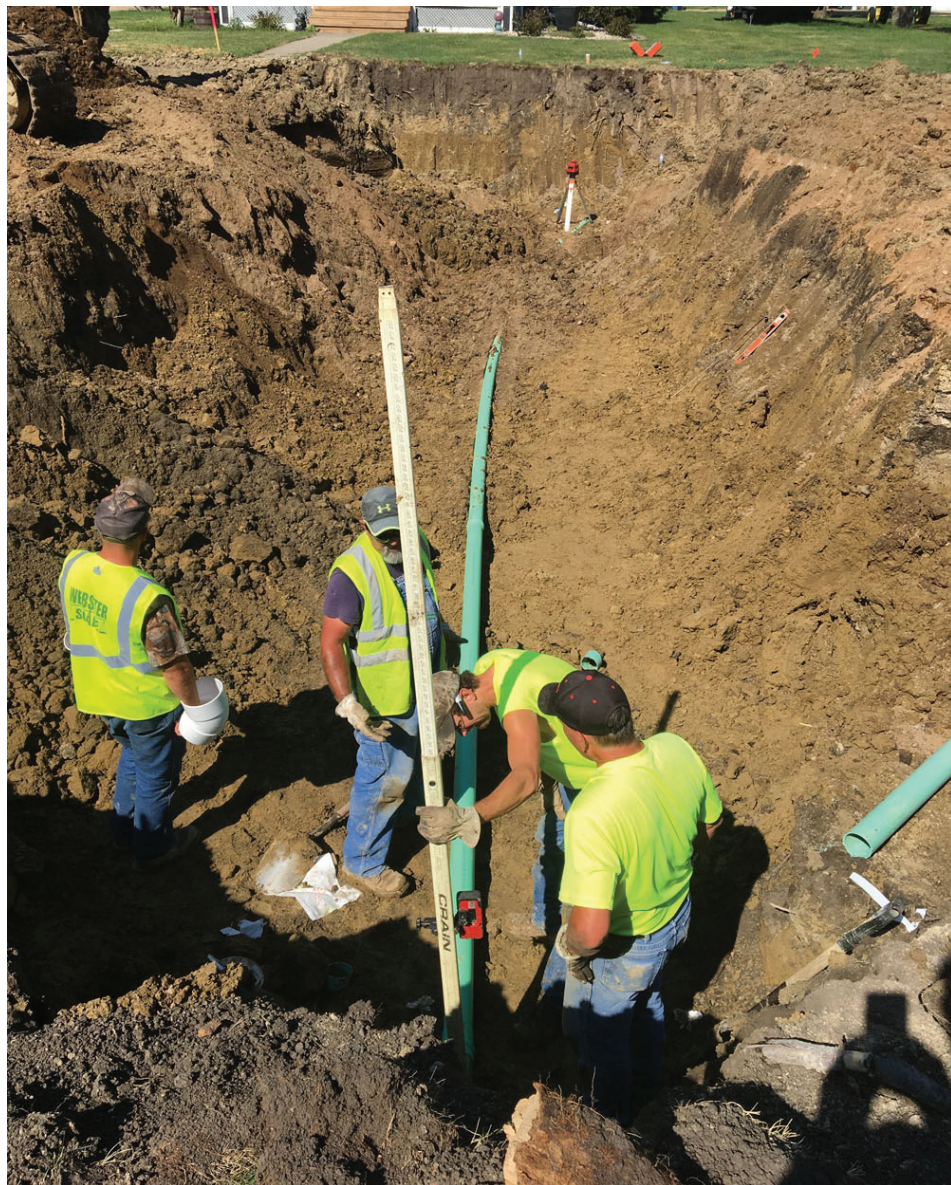
City employees Dwight Zerr, Branden Abeln and Terry Heron were installing the new sewer service line for one of the homeowners. Four services had to be lowered and it is now known yet if a fifth service line will have to be lowered. Also pictured on the left is an employee of Webster Scale.
