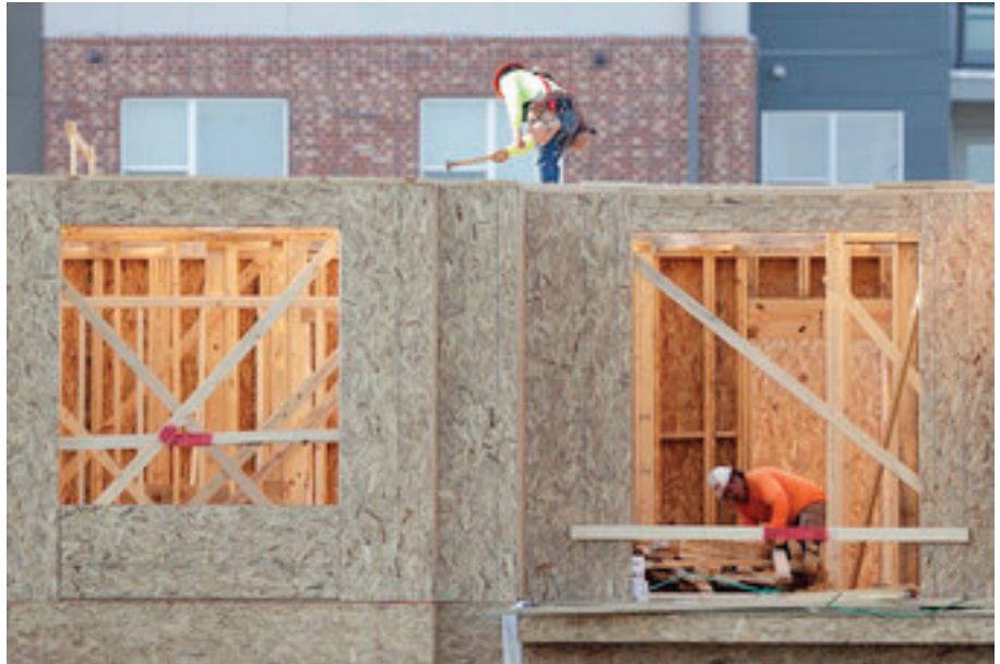
In this July 12, 2017, photo, construction workers build a residential complex in Nashville, Tenn. On Friday, July 28, 2017, the Commerce Department issues an economic report on how the U.S. economy is performing. (AP Photo/Mark Humphrey)
