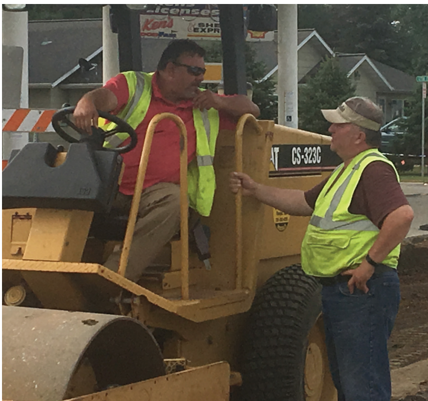
John Shoemaker (right) of Webster Scale is talking with one of his employees, Mo. Mo is on the packer getting the sidewalk and curb ready on Saturday so it can be poured on Monday.
