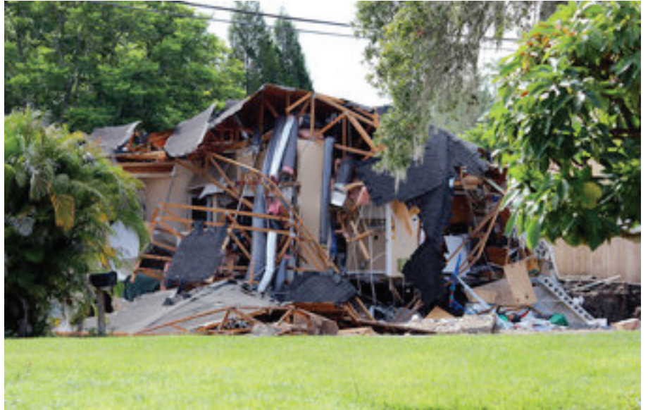
Debris is strewn about from a partially collapsed home in Land O' Lakes, Fla. on Friday, July 14, 2017. A sinkhole that started out the size of a small swimming pool and continued to grow has swallowed a home in Florida and severely damaged another. (Alessandra da Pra/Tampa Bay Times via AP)
