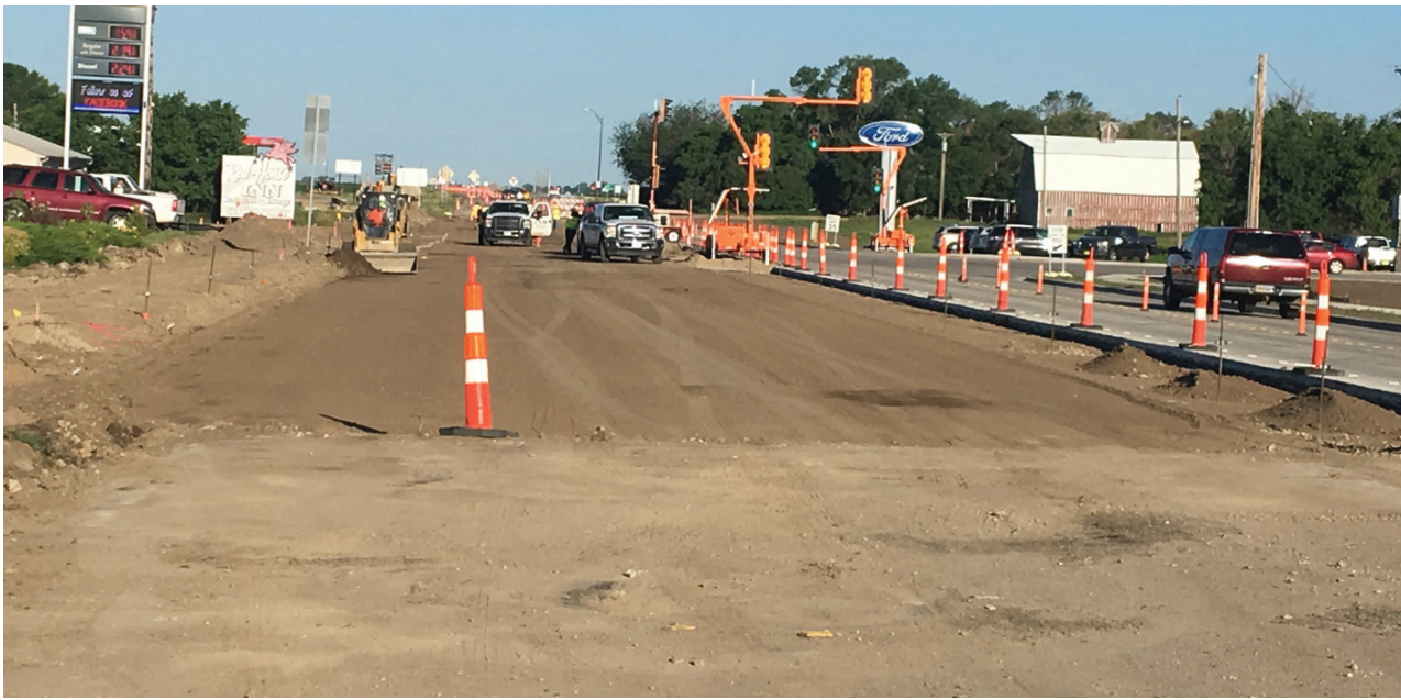
Crews were busy working on the south lane of US 12 in Groton Saturday morning. They are trying to get everything done so it can be poured by Thursday of this upcoming week. (Photo by Paul Kosel)
