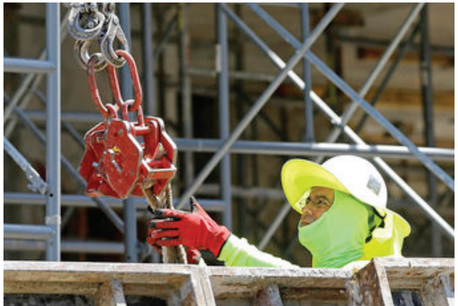
In this Thursday, June 15, 2017, photo, a construction worker continues work on a condominium project in Coral Gables, Fla. On Friday, July 7, 2017, the Labor Department will release the U.S. jobs report for June. (AP Photo/Alan Diaz)
