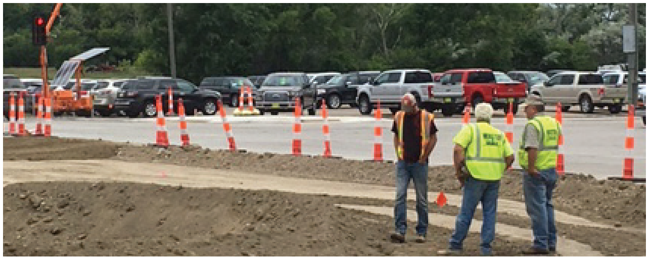
Work continues on the US12 project in Groton as Webster Scale, Inc. employees take a look at the progress. The new completion date for US12 is now July 28th. The set-back from the July 1 deadline is mainly because of utility conflicts, according to the weekly DOT report held yesterday. (Photo by Tina Kosel)
