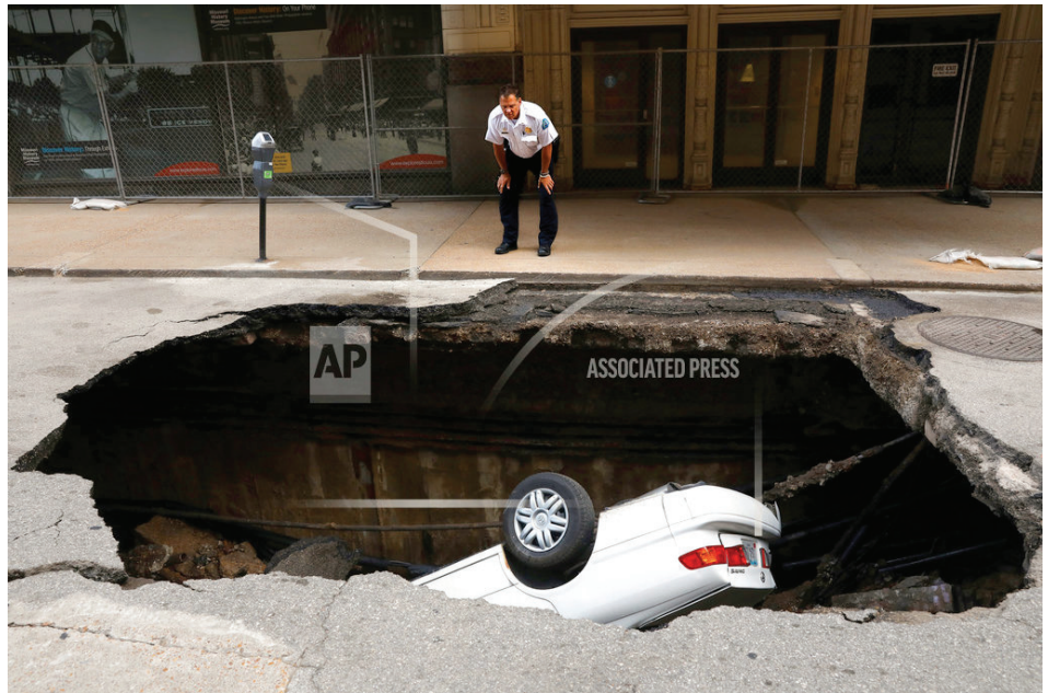
A St. Louis police officer looks over a large hole in 6th Street, Thursday, June 29, 2017, in St. Louis, that swallowed a Toyota Camry between Olive and Locust Streets. It isn't immediately clear what caused the collapse. (Christian Gooden/St. Louis Post-Dispatch via AP)
