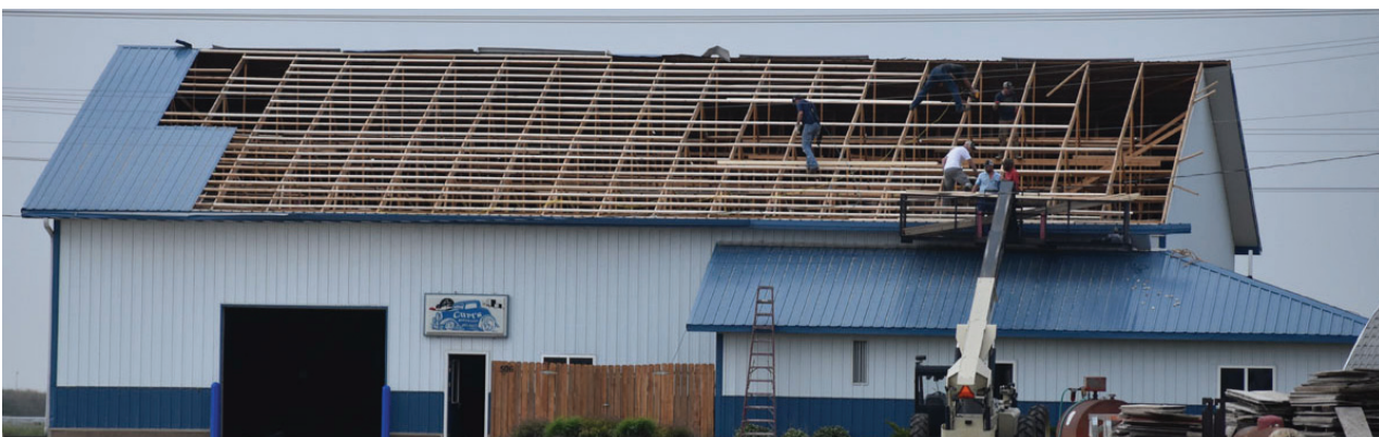
Several workers were working as fast as they could to reinforce the roof before the next round of storms would come through the area Tuesday evening. (Photo by Paul Kosel)
