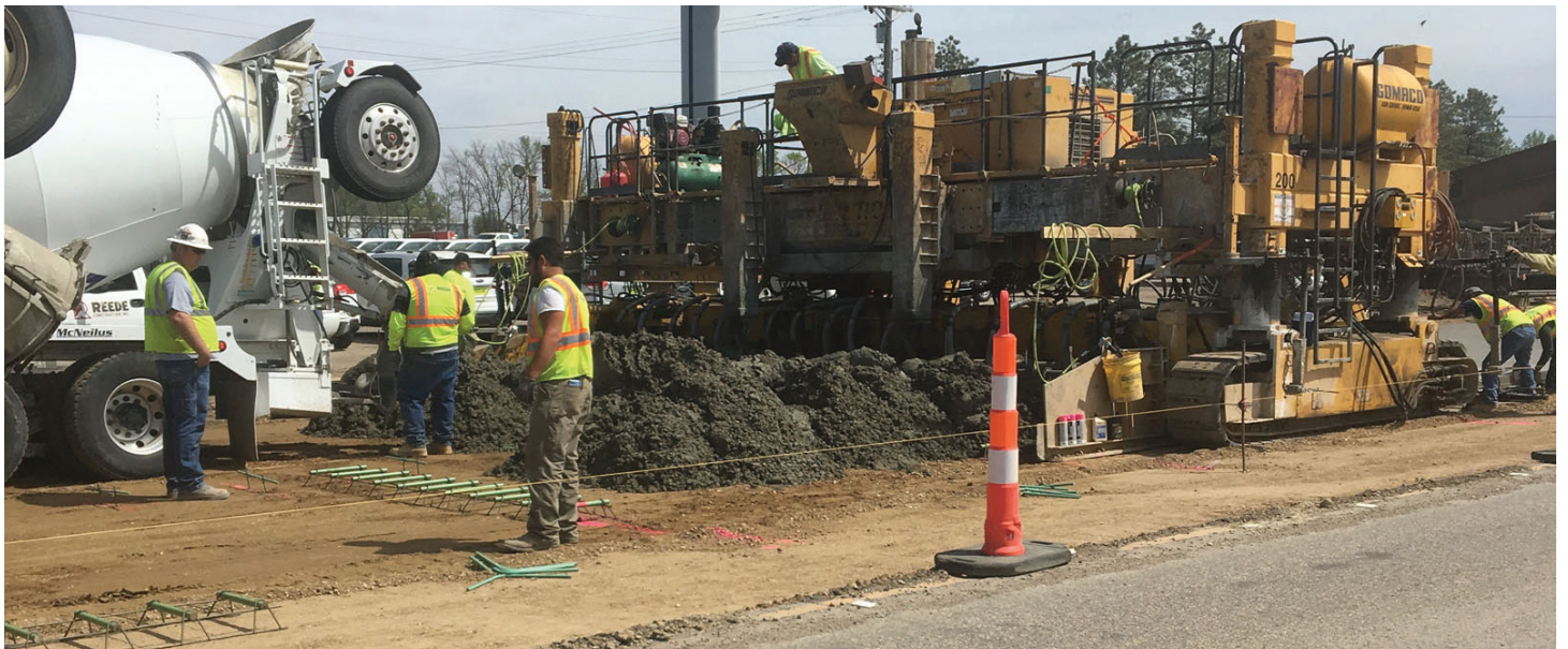
More concrete was laid down on the US12 project. This time on the west side of the project.
