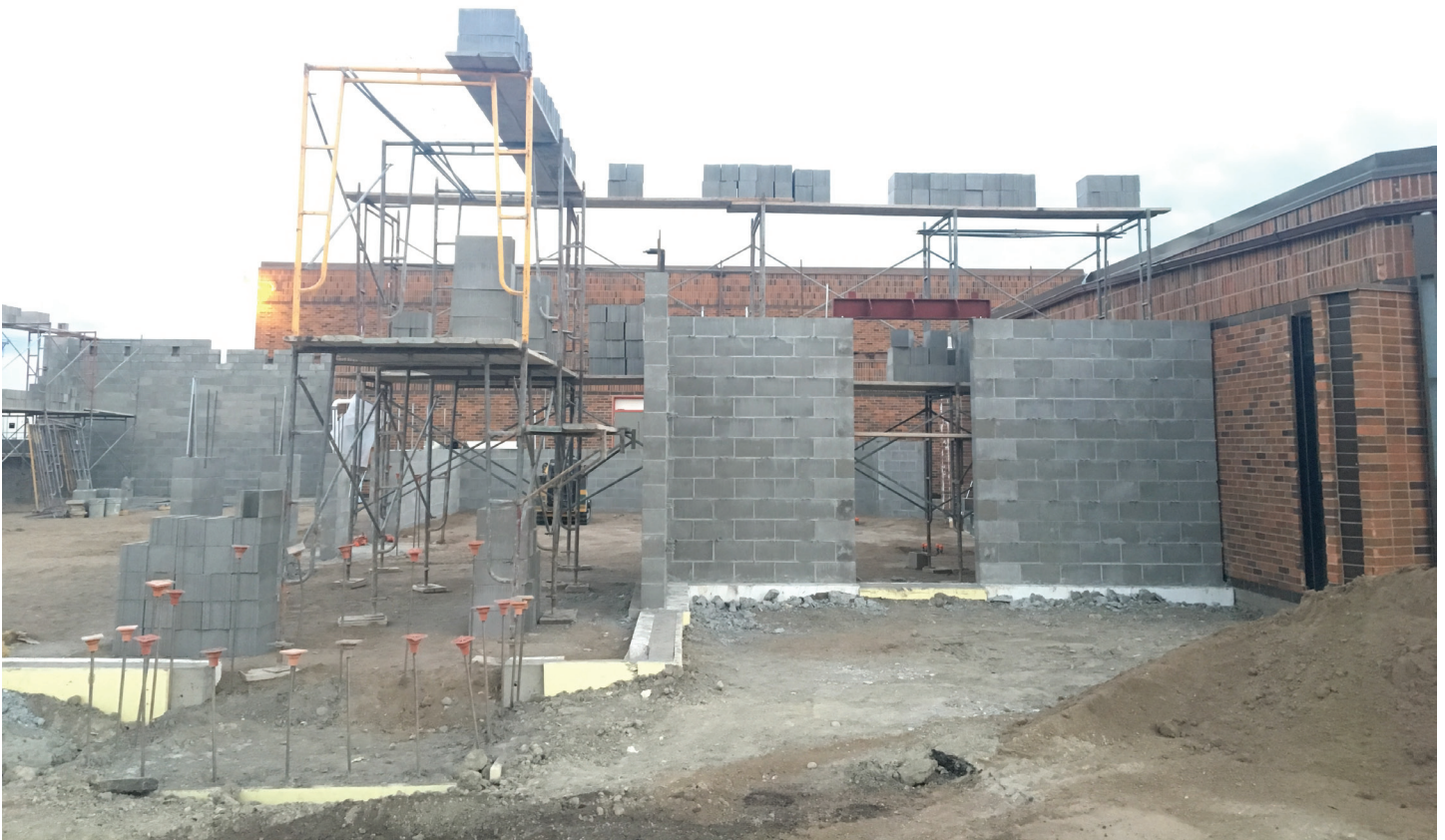
The brick work is progressing on the new addition to the Groton Area Elementary School. The new addition will serve as the new lunchroom, freeing up the gym.
