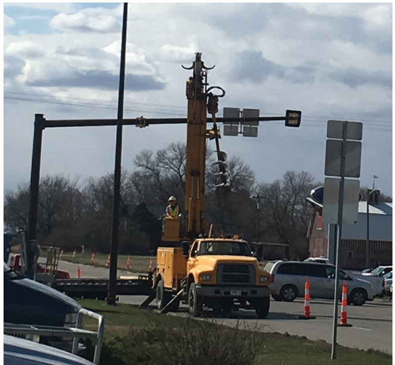
The old flashing lights were taken down yesterday as work on US12 in Groton begins.
