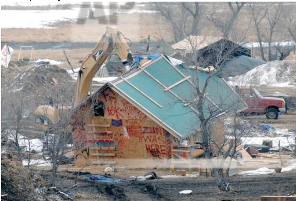
A backhoe rips through a wood structure to begin the cleaning up process at the Oceti Sakowin camp as law enforcement swept through the camp arresting the final Dakota Access oil pipeline protesters in Morton County Thursday, Feb. 23, 2017, near Cannon Ball, N.D. (Mike McCleary/The Bismarck Tribune via AP, Pool)
