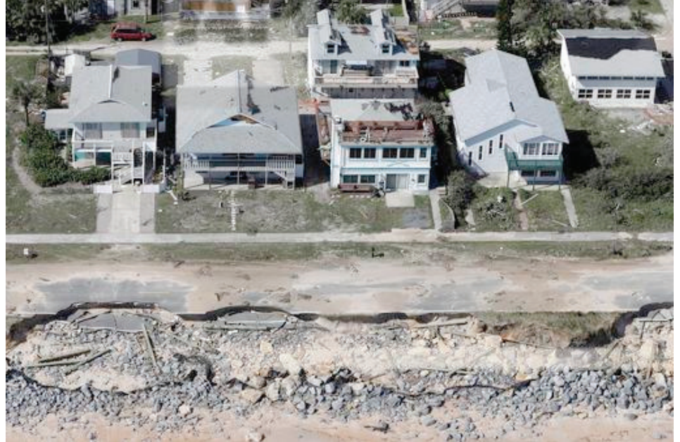
In this aerial photo, portions of SR A1A are washed out from Hurricane Matthew, Saturday, Oct. 8, 2016, in Flagler Beach, Fla. The damage from Matthew caused beach erosion, washed out some roads and knocked out power for more than 1 million customers in several coastal counties. (AP Photo/Chris O'Meara)
