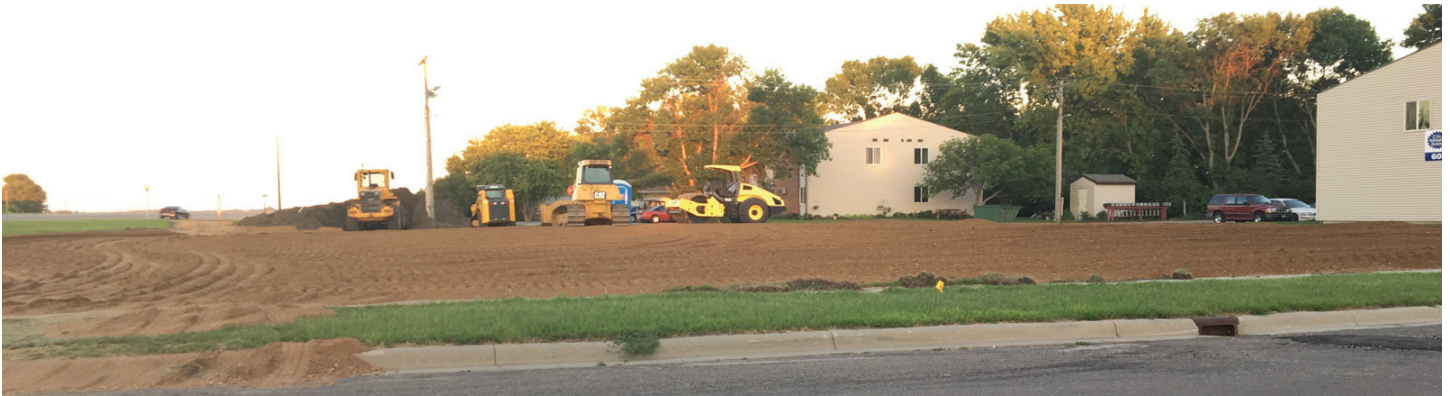
The gravel was put down on the site of the new Dollar General Store on Tuesday.
