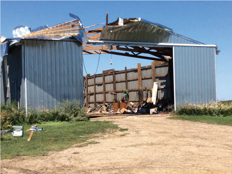
Roof removed from an outbuilding 3 miles west-northwest of Bristol
