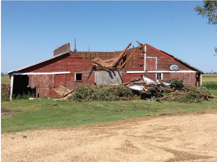
Damage to a barn located 1 mile east of Andover
