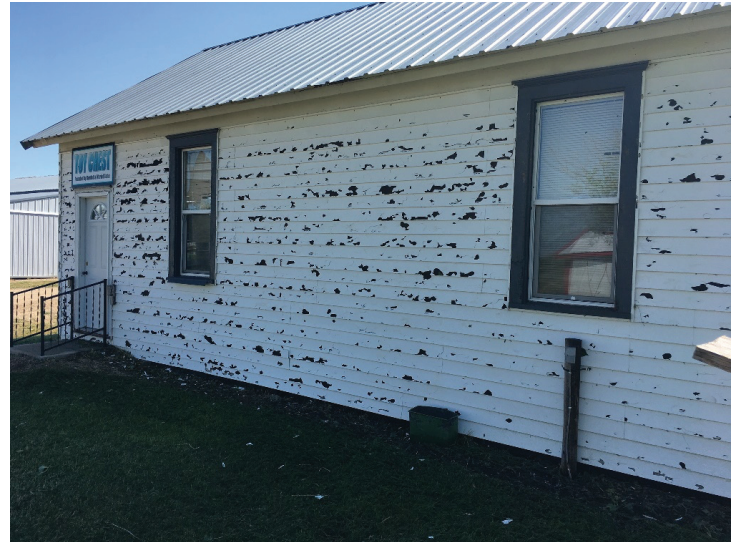
One of the several buildings in Threshermen's Park in Andover that were damaged by hail.
