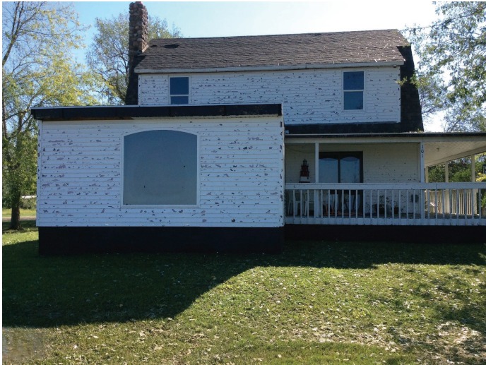
Wind driven hail damage to a house on the west side of Andover
