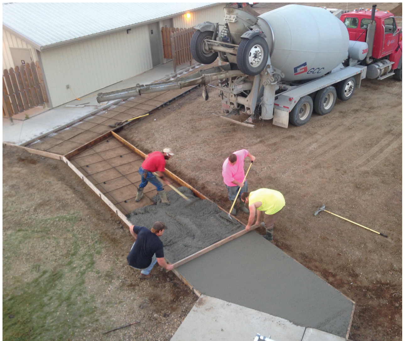
The new sidewalk was being poured this morning between the bathrooms and the bleachers. Pictured are Joe Foertsch in red, Nick Olson in pink, Justin Olson in yellow and Jeff Krueger in black.
