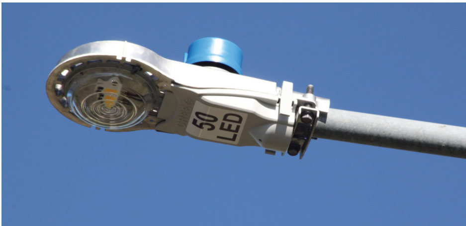
These are new LED lights that are being installed throughout town.
