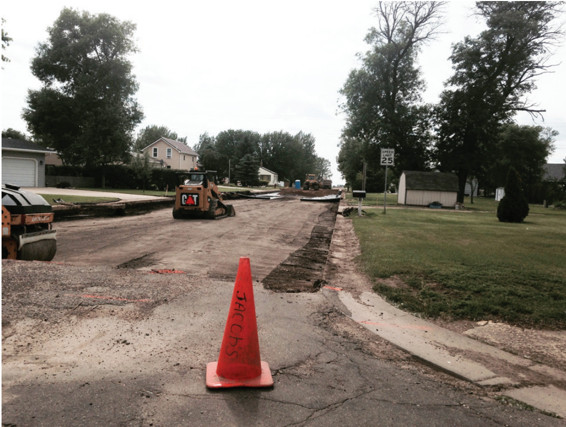
Road construction of Fifth Avenue West continues as they near the end of the project.
