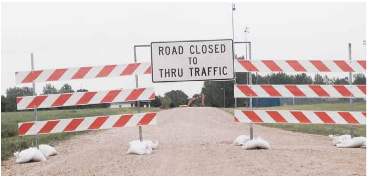
Construction has begun on the Fifth Avenue West project. The construction area is starting on the west edge and will head east. They are currently just west of Garfield Street on West Fifth Avenue.
