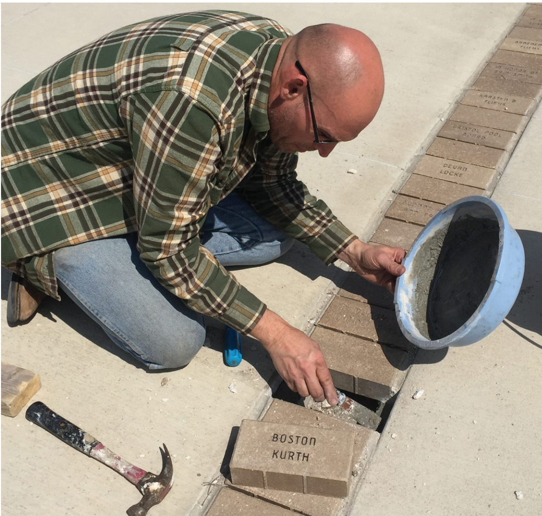
Paul Kosel was installing two new bricks at the Groton Swimming Pool on Thursday. Bricks for Jody Opp and Boston Kurth were installed. There is still time to get your brick for this season. Contact City Hall at 397-8422 to order your brick. (Photo by Justin Olson)
