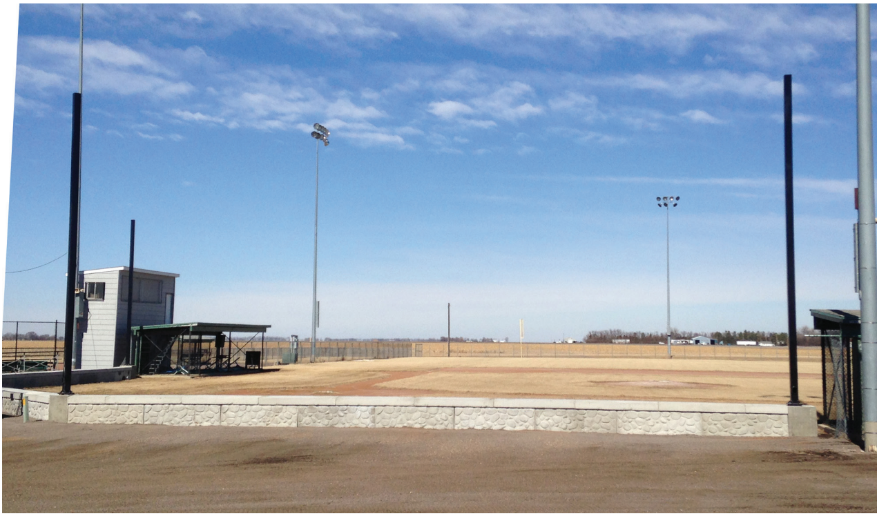
The work on the concrete backstop was completed Friday by employees of the city.
