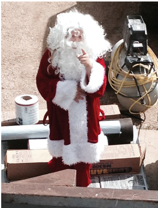
Santa even paid us a visit while we were shingling the roof. He was not happy when we permanently removed a chimney. Cute Jeslyn.
