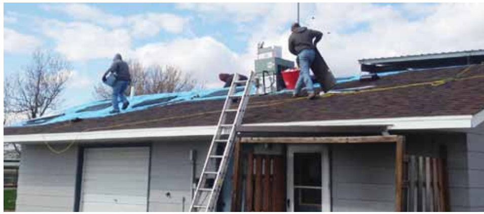
The crew from Blocker Construction donated their time to reshingle the roof of the concession stand at the Groton Baseball Complex. The work was done last week.
