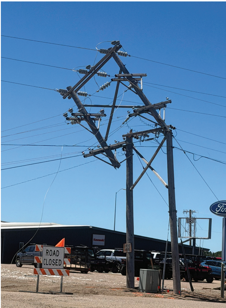
There was nothing left of the electrical infrastructure in Highmore after the storm on Monday. (Photo by Paul Kosel)
