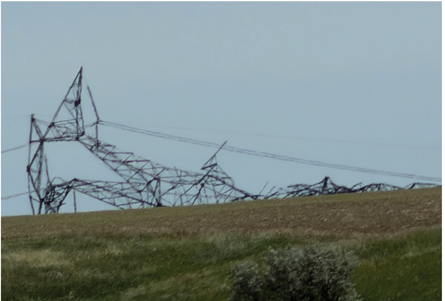
Transmission line towers were destroyed by the strong wind 13 miles north of Miller from the storm that went through the area on Monday. (Photo by Paul Kosel)
