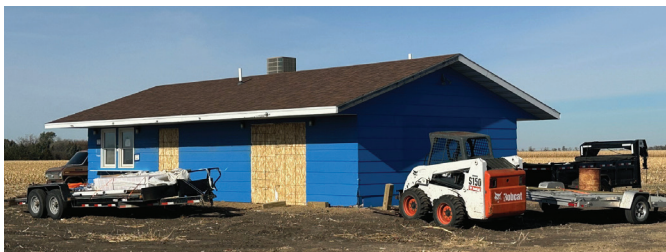
The former baseball concession stand has a new home at the Groton Municipal Airport. It will be converted into a Pilot's Lounge.
