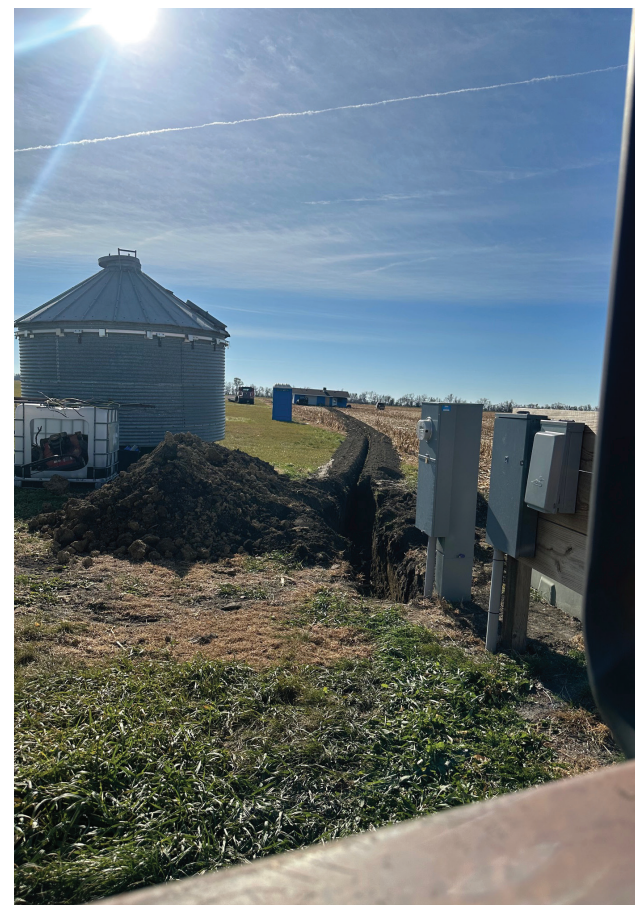
A 500' trench was done to provide power to the Pilot's Lounge; however, the distance of 500 feet is too far and would cost over $5,000 to install secondary wire, while adding a second transformer would cost roughly the same amount.
