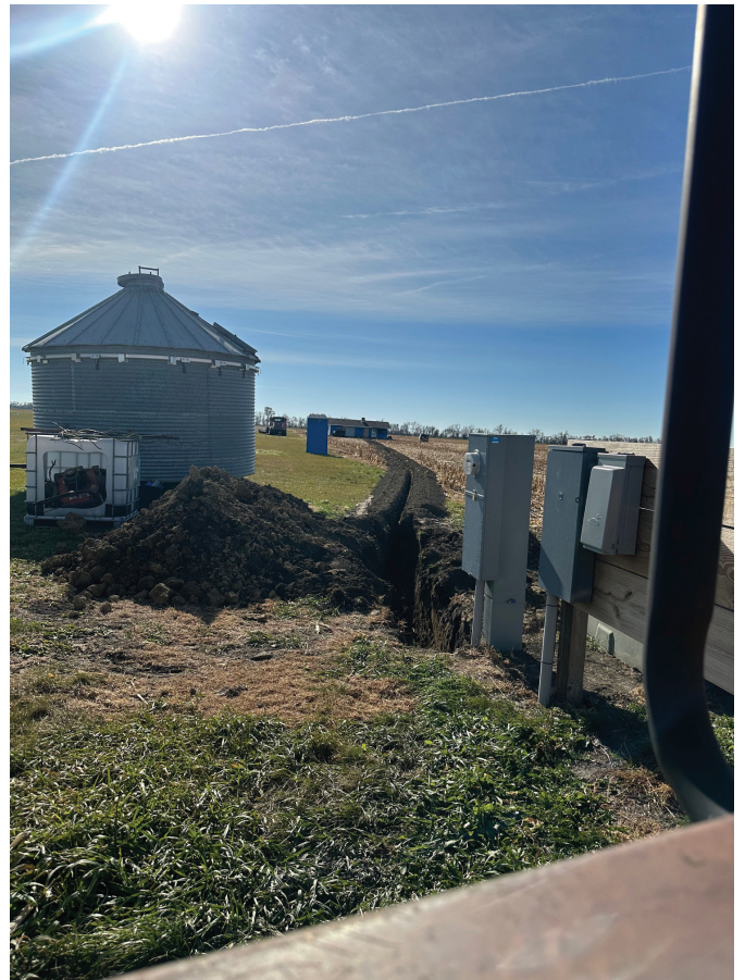
A 500' trench was done to provide power to the Pilot's Lounge; however, the distance of 500 feet is too far and would cost over $5,000 to install secondary wire, while adding a second transformer would cost roughly the same amount.
