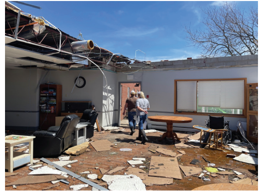
The dining room at the Avantara Nursing Home in Salem, S.D., on May 13, 2022, one day after a derecho wind storm severely damaged the structure. (Photo: Annie Todd/Sioux Falls Argus Leader)
