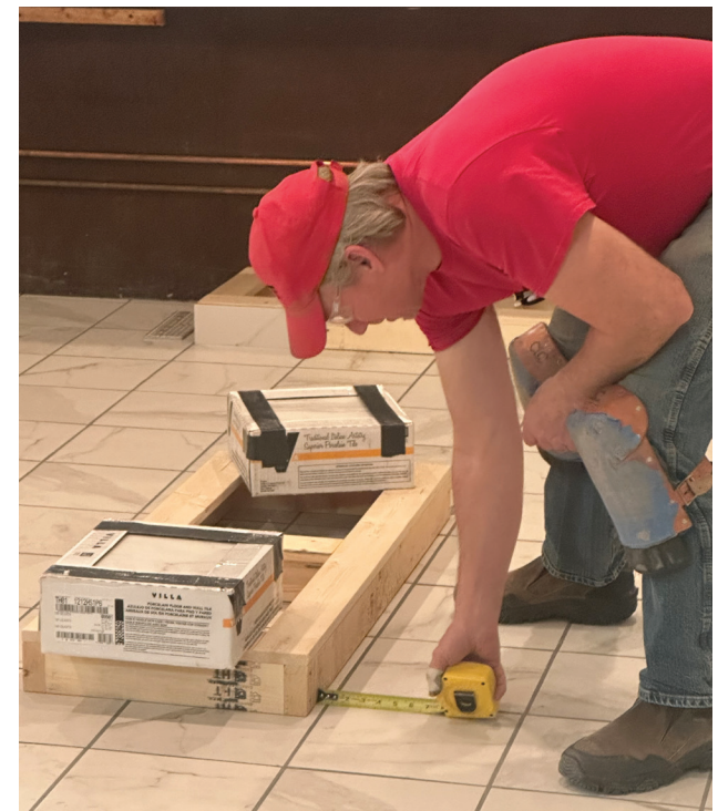
John Sippel is measuring for the placement of the bar stand area. (Photo by Paul Kosel)
