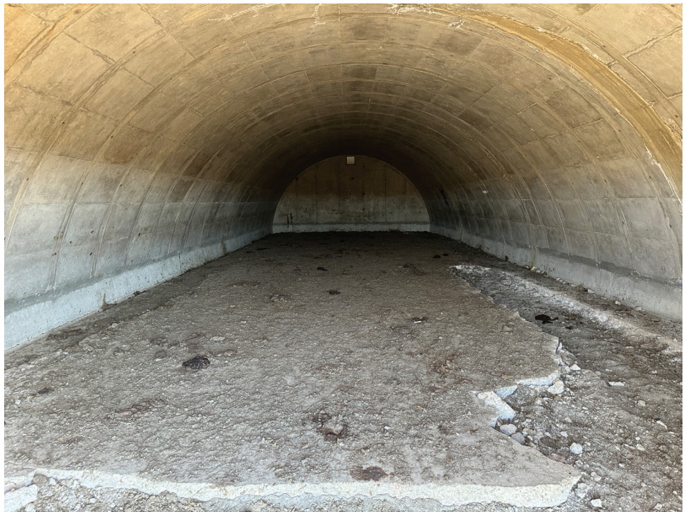
This photo, taken on Oct. 4, 2024 at the Vivos xPoint bunker complex near Igloo, S.D., shows an empty bunker before any improvements are made. (Photo: Bart Pfankuch / South Dakota News Watch)
