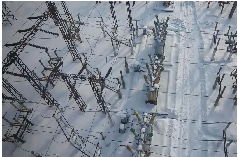
An electrical substation in the snow in winter.
