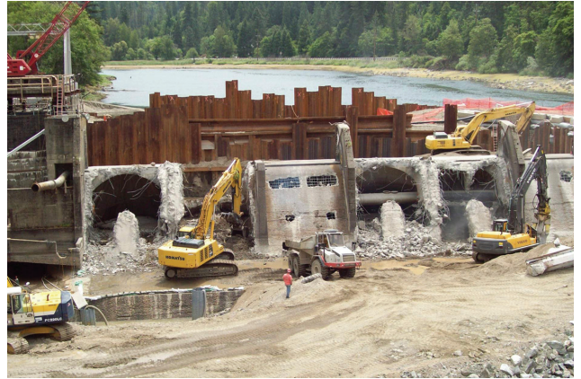
Workers dismantle the Savage Rapids Dam on the Rogue River in Oregon. Credit: Oregon State University, FlickrCC.
