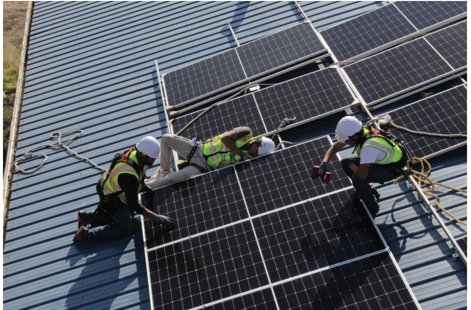
Lightspring Solar apprentices install solar panels on the roof of a community building in the small township of Wakpala, on the Standing Rock Reservation. (Grace Fiori/Buffalo's Fire)
