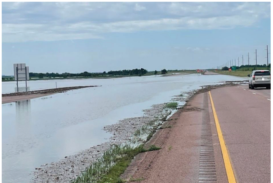
A flooded southeast South Dakota road on June 21, 2024.
