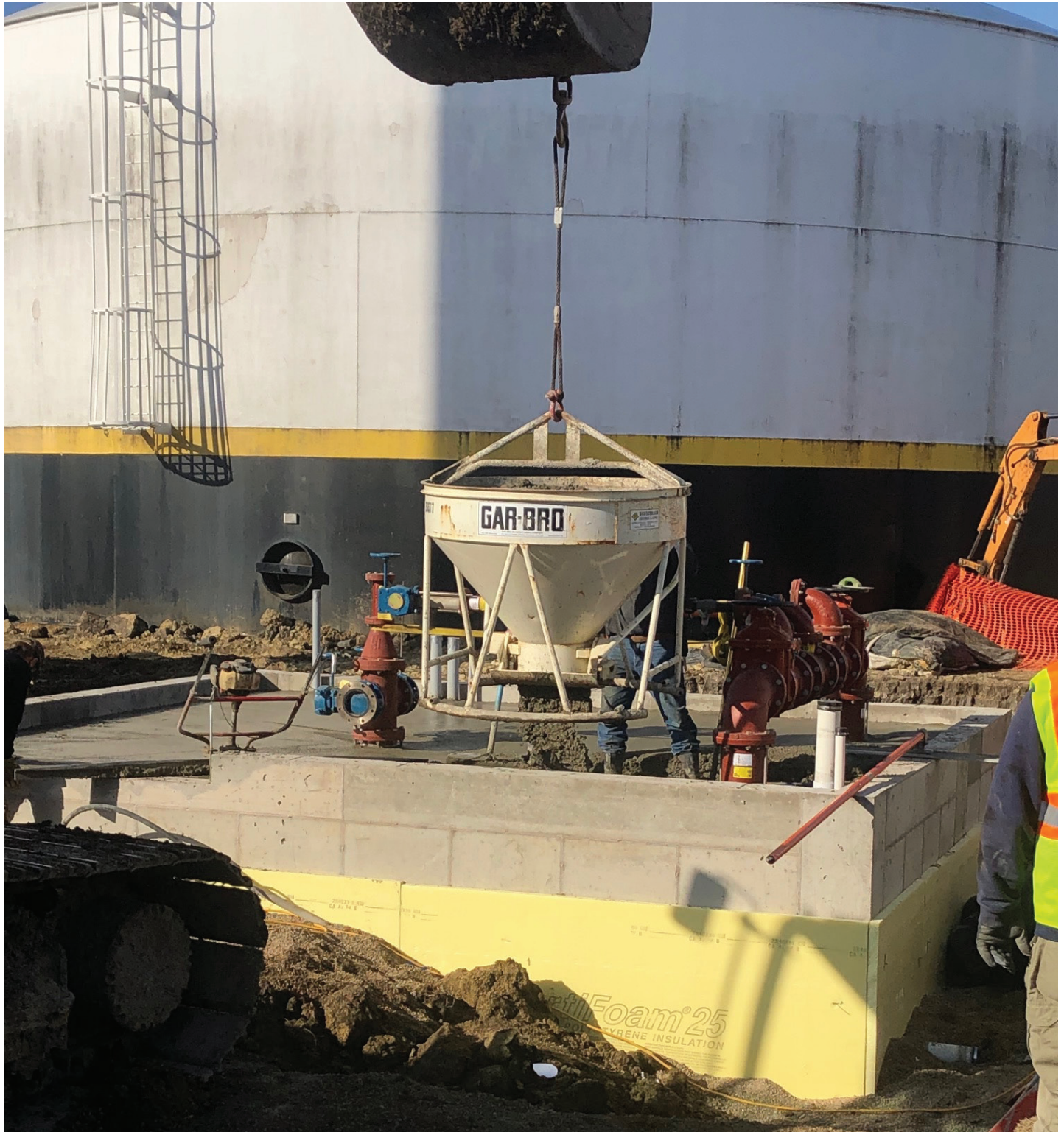
Concrete was lowered down in this carrying device and then released. The floor for the new pump room was poured on Thursday. (Photo by Paul Kosel)
